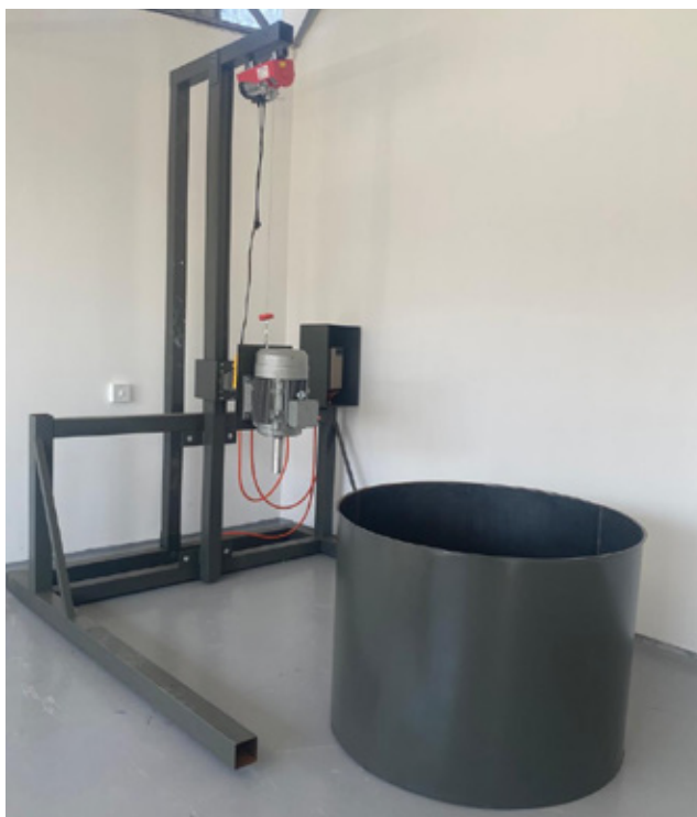
Detergent manufacturing equipment procured and installed at Vula Detergents Share Manufacturing Facility in Madadeni
